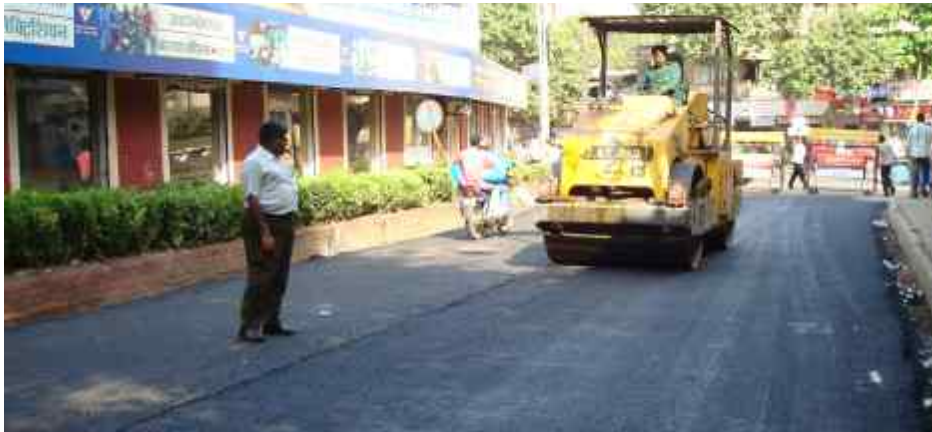
MCGM is constructing an Asphalt Road with about 15% Plastic Wastes near Dadar Station in Mumbai (Prof. V. S. Agashe Road) with technical assistance from ICPE.
